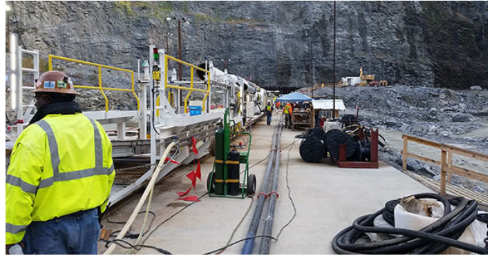
Trailing gear of TBM, Bellwood Quarry, Atlanta, Georgia. Credit: R. Kath, 2015
