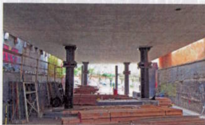
LATERAL SYSTEM Ground-floor pipe columns, with isolators, span vertically between grade beams and the second-floor slab of the three-story building.
