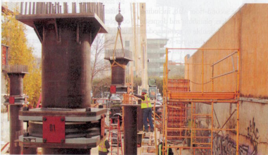
COLUMN MOUNTED A system of triple-pendulum bearings spliced into columns cost less than base isolators because there is no excavation required for a basement level.
